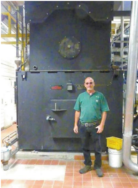
Ventilation and refrigeration technician Gary Roberts runs the wood boiler system at National Life in Montpelier. PHOTOS BY PETER COBB
